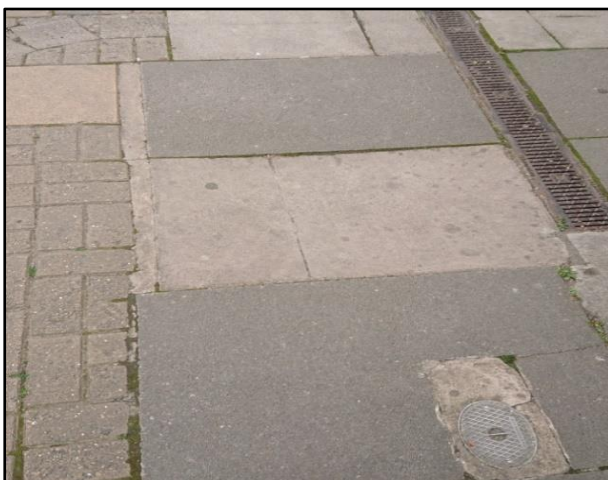
Poor paving and reinstatement, Leicester Road.
