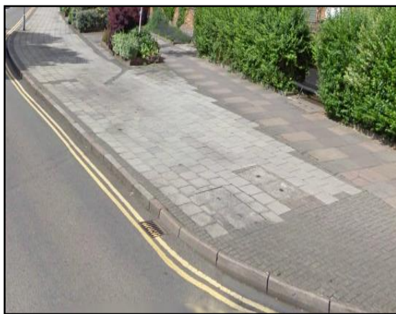
Illustrations of the number of surfacing materials used and the general condition
